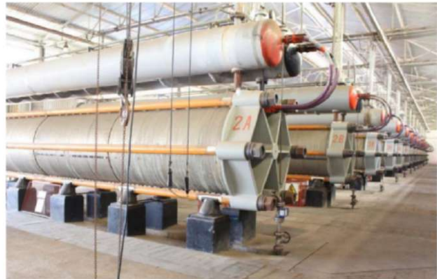
Situation in 2017... the plant (128MVA) has been shut down end 2015... after operating for 45 years
