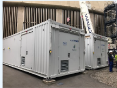
ALIGN-CCUS water electrolysis system (Niederaussem, Germany)
