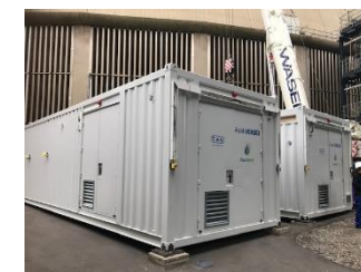
ALIGN-CCUS Water electrolysis system (Niederraussem, Germany)
