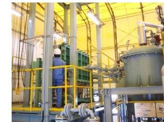
Souma IHI green energy center Alkaline water electrolysis system
