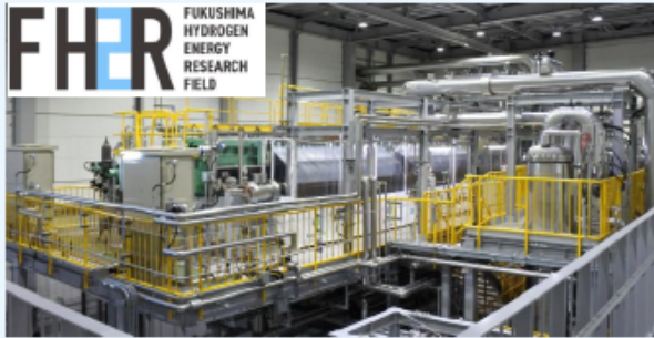
NEDO project Fukushima Hydrogen Energy Research Field (FH2R)
